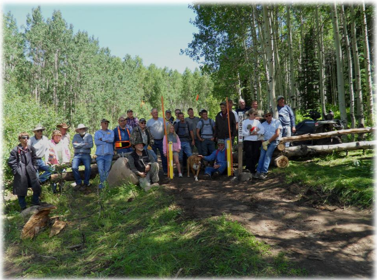
Above is width restrictor and log fencing installed on the west end of High Trail. The Orange marker posts are so snowmobile users will see the location.
