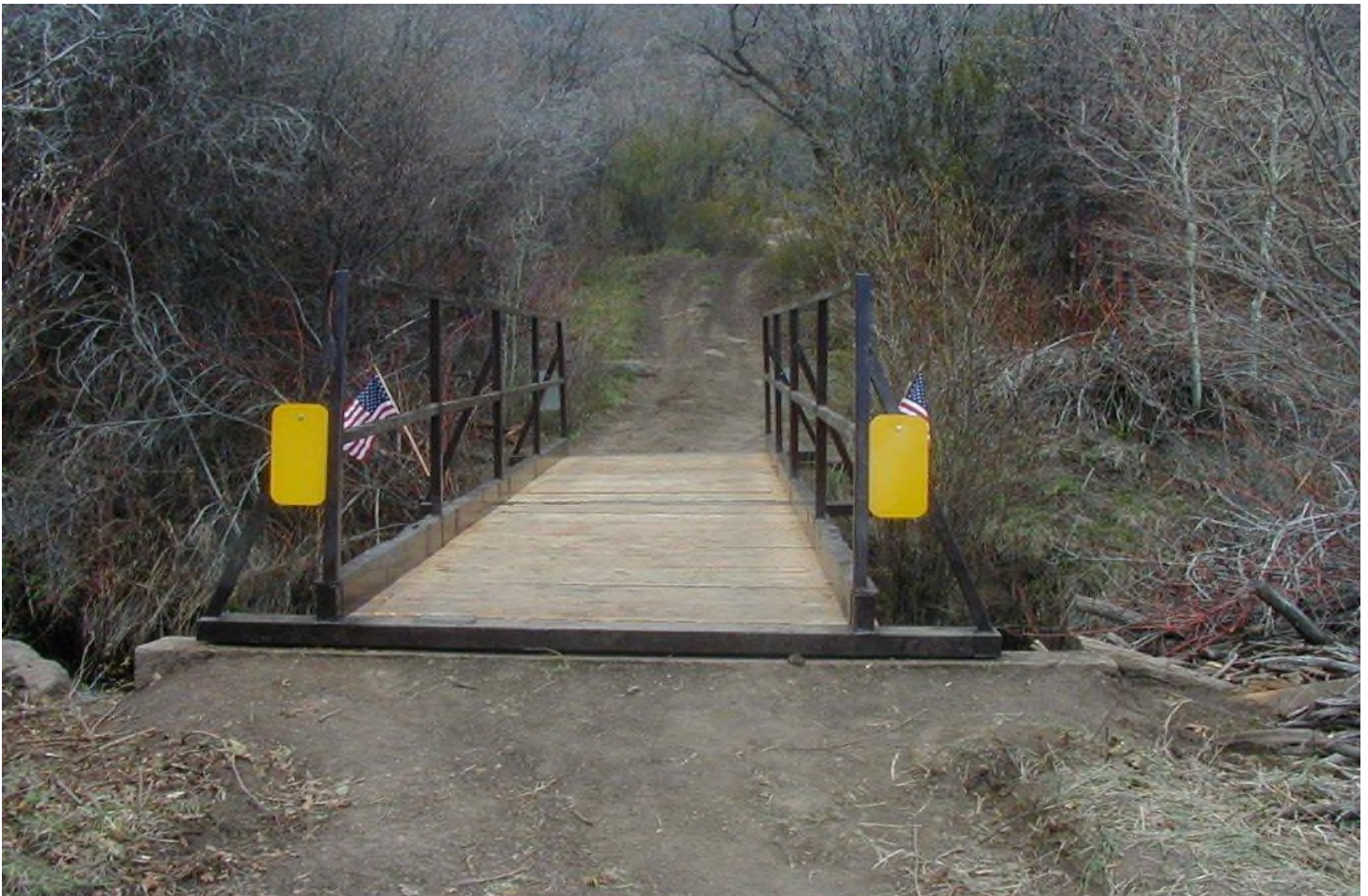
The completed bridge, with American flags in place to signify it was made in America.
